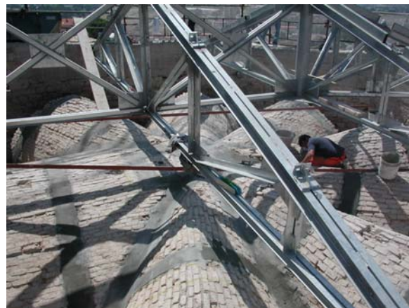
Retrofit job of the vaults using carbon fiber sheets and steel roof structure
